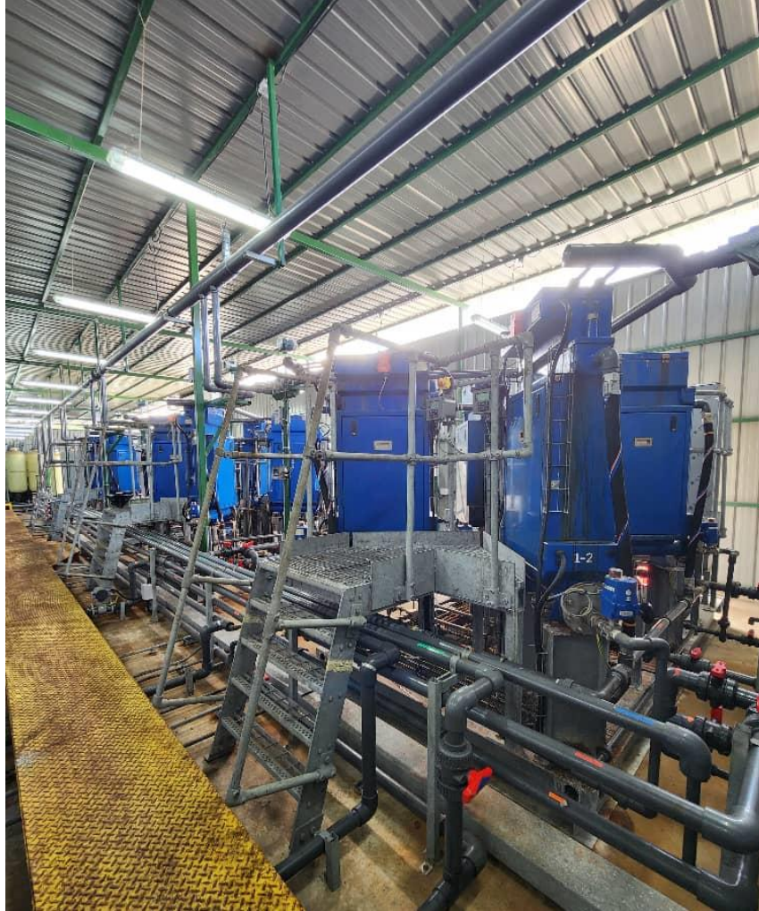
ICM's pilot plant facility in Singapore
