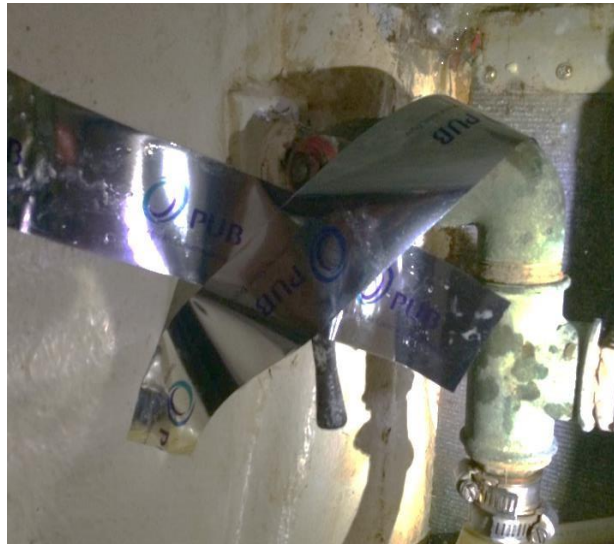
Photo of PUB secondary seal over a 'Y' valve
